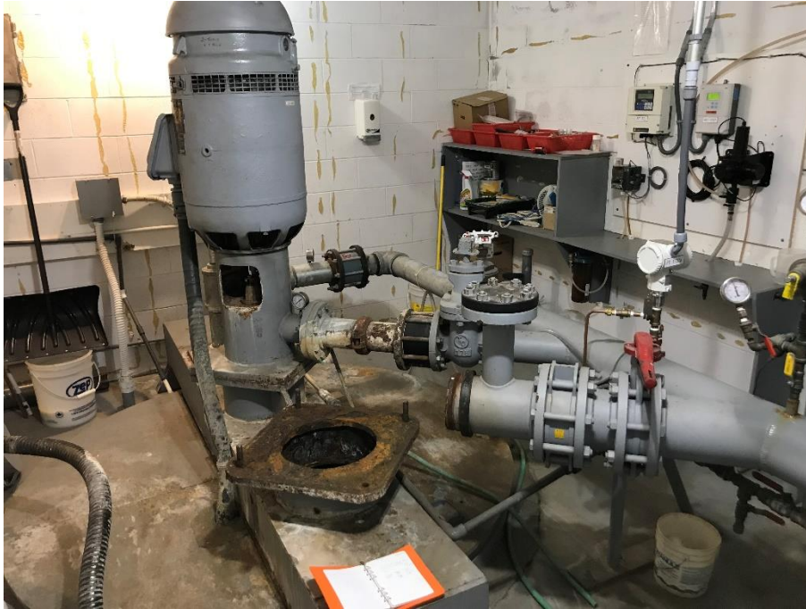
Figure 2: View of pump pedestal with heaviest vertical turbine (in foreground) removed
